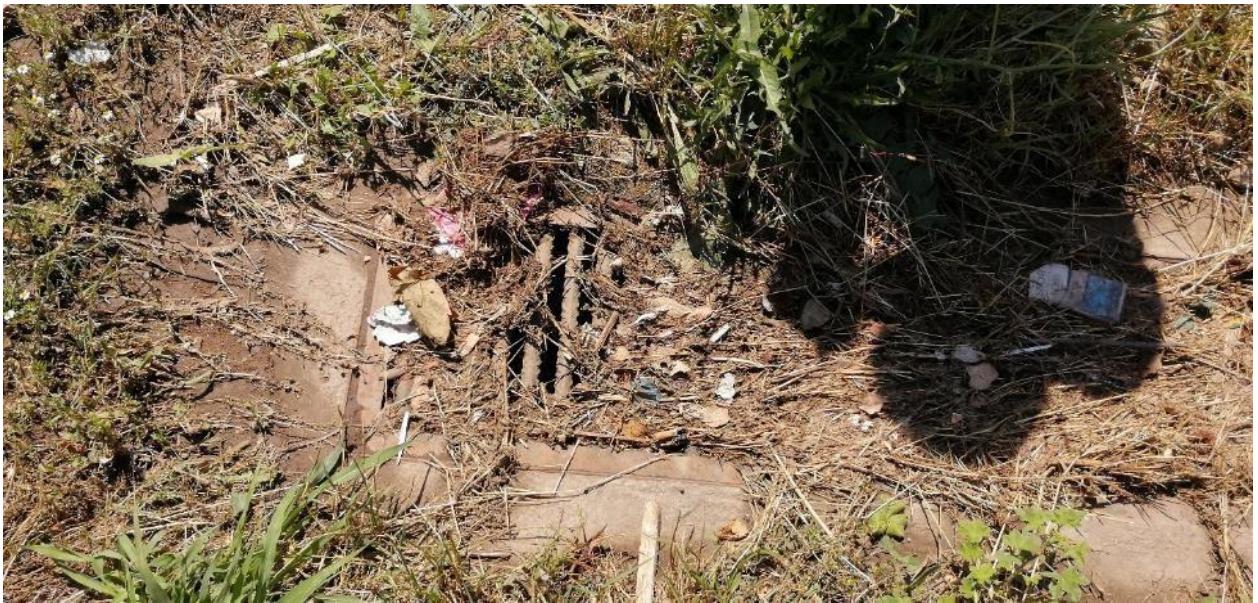
19. Figure: Clogged gully pot
