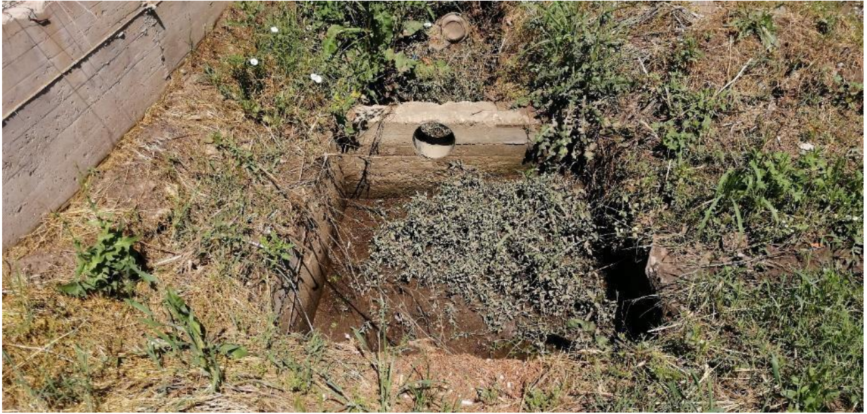
20. Figure: Unusable drainage element
