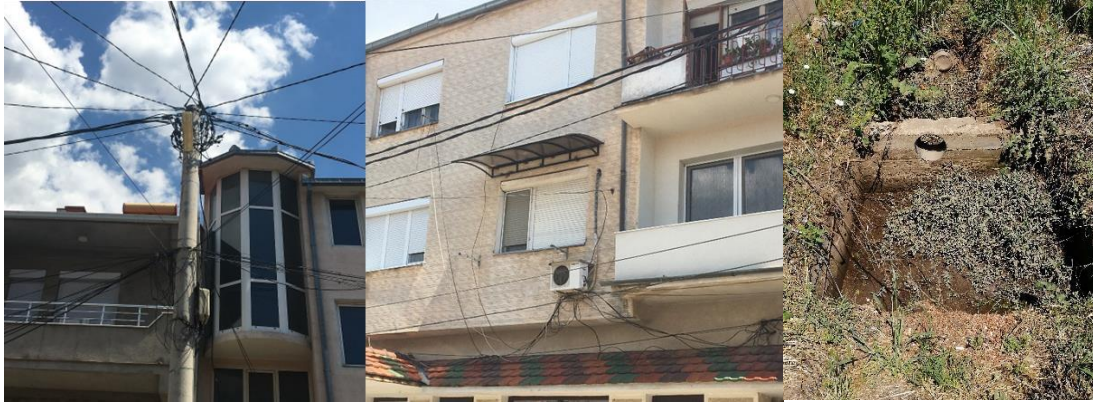
1. Figure Vulnerable electric infrastructure and drainage system pieces in Vinica, North Macedonia.
